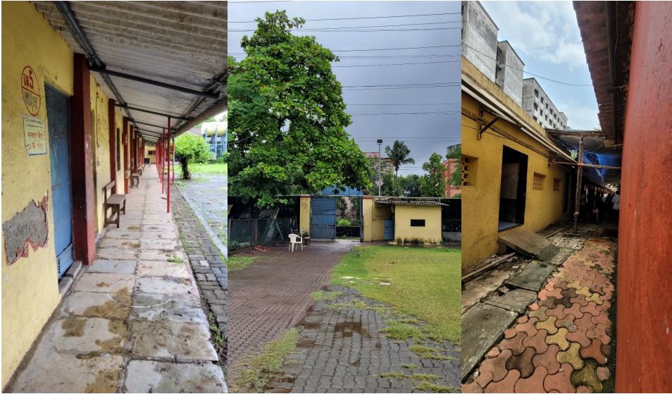
Figure 3. Corridor with a metal shed, an uneven pathway to the entrance gate, and a washroom with ramped access. Source: Author
